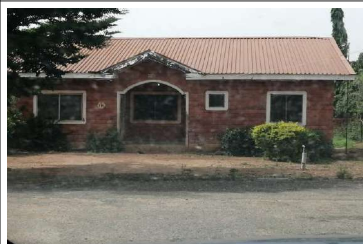
Plate 4: Another low-income scheme located on the outskirts along Suleja road. This scheme is fairly decent when compared to most of the low-income schemes with the provision of some infrastructure. However, it is poor maintained and is in a dilapidated state
