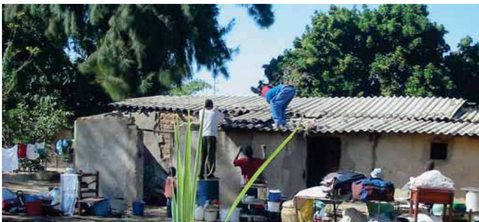
Figure 25: A family repairing the roof of their house in Zimbabwe. Photo © UN-HABITAT
