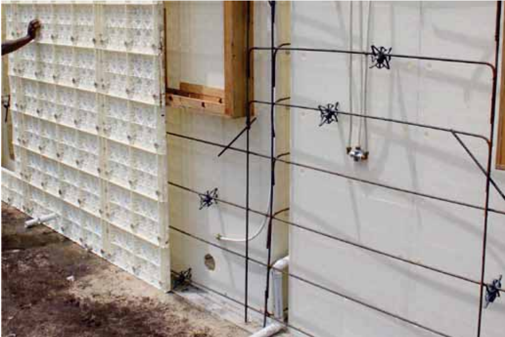
Figure 26: An exposed wall cavity of a Moladi house prior to casting. Photo © Camalynne Botes/Moladi
