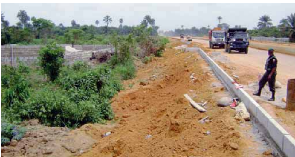
Figure 18: Laying infrastructure in anticipation of urban development, Nigeria. Photo © UN-HABITAT/ Claudio Acioly
