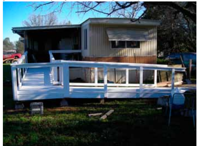
SHHIP installs items like this ADA compliant ramp which allows the resident safe and easy access to the home.
