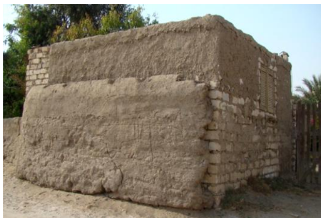
Figure 23: Attempts to add a layer of mud brick or plastering to the exterior limestone walls for improving thermal comfort.
