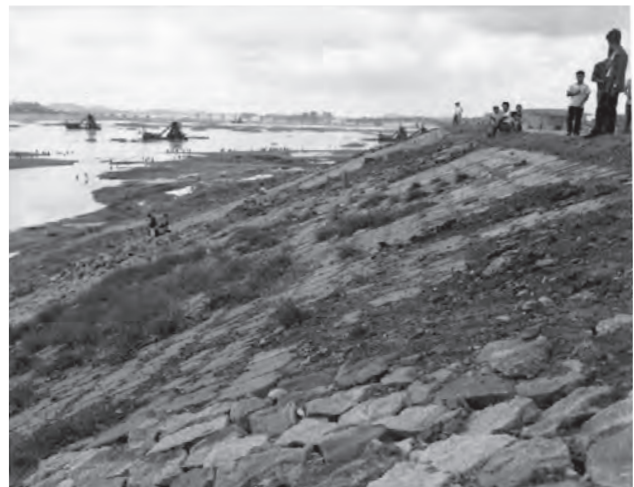
Figure 3-9. New embankment on the northern side of the Han River. Photograph taken in Hannam-dong, 1967. The Hannam bridge is being built in the background. Source: Seoul Museum of History (서울역사박물관).
