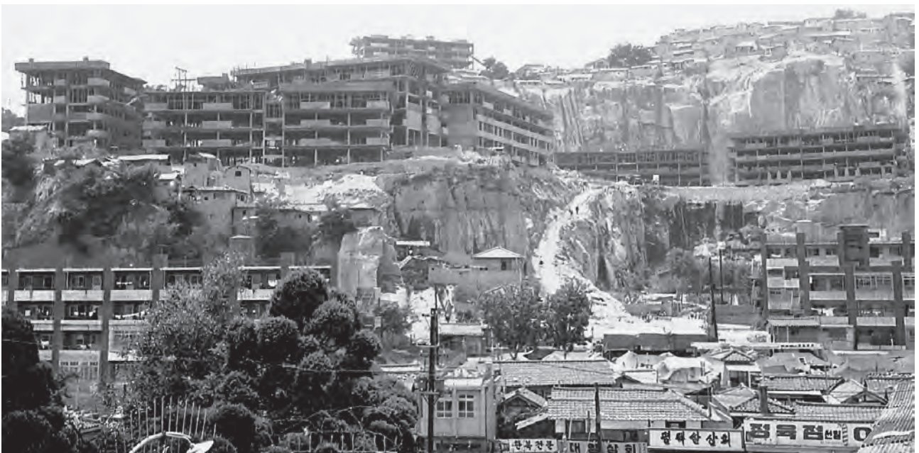
Figure 3-24. Naksan apartments, 1969. Buildings under construction on the site of former informal settlements accopying the quarries of Changsin-dong. The apartments were demolished in 1998 due to safety and scenic issues. Source: Seoul Museum of History (서울역사박물관).
