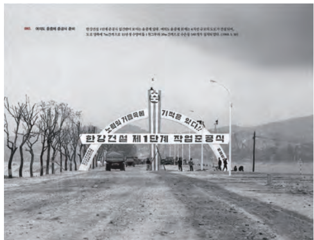
Figure 3-10. Construction of a four-lane road on the embankment along the river. Yeouido Island, 1968. Source: Seoul Museum of History (서울역사박물관).
