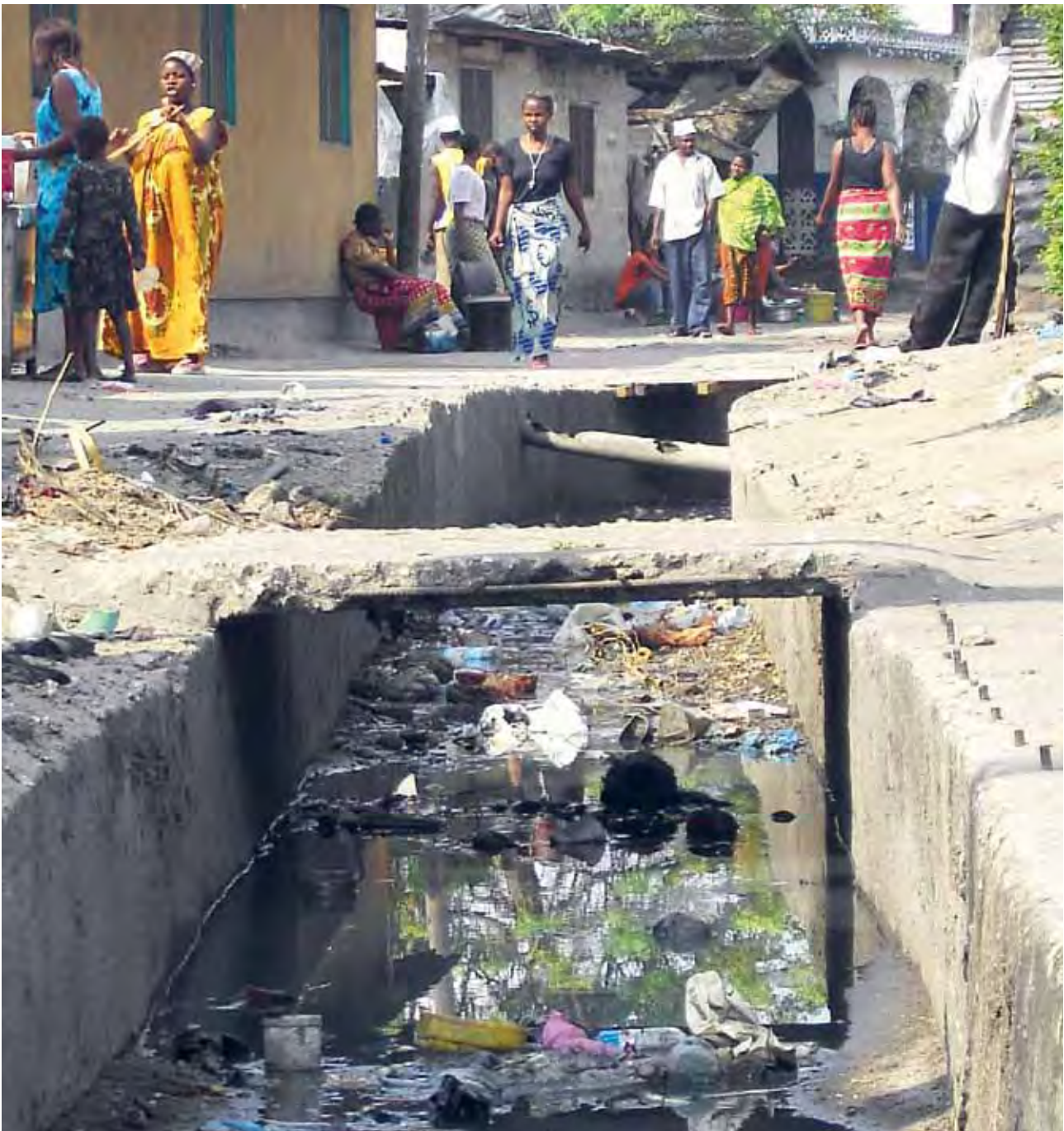
Open drainage in Hanna Nassif, constructed during community-based settlement upgrading (1990-94) Photo © Rasmus Precht
