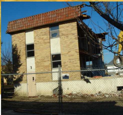
Demolition of vacant St. Peter’s convent makes way for affordable housing - Pleasantville, NJ
