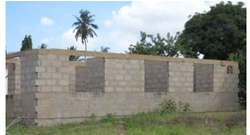
Houses stand uncompleted for many years. If prices could have been estimated more accurately, the owner could have completed a modest, but habitable house. As it is, completing the house is beyond his means. (Makangarawe, Dar es Salaam)
