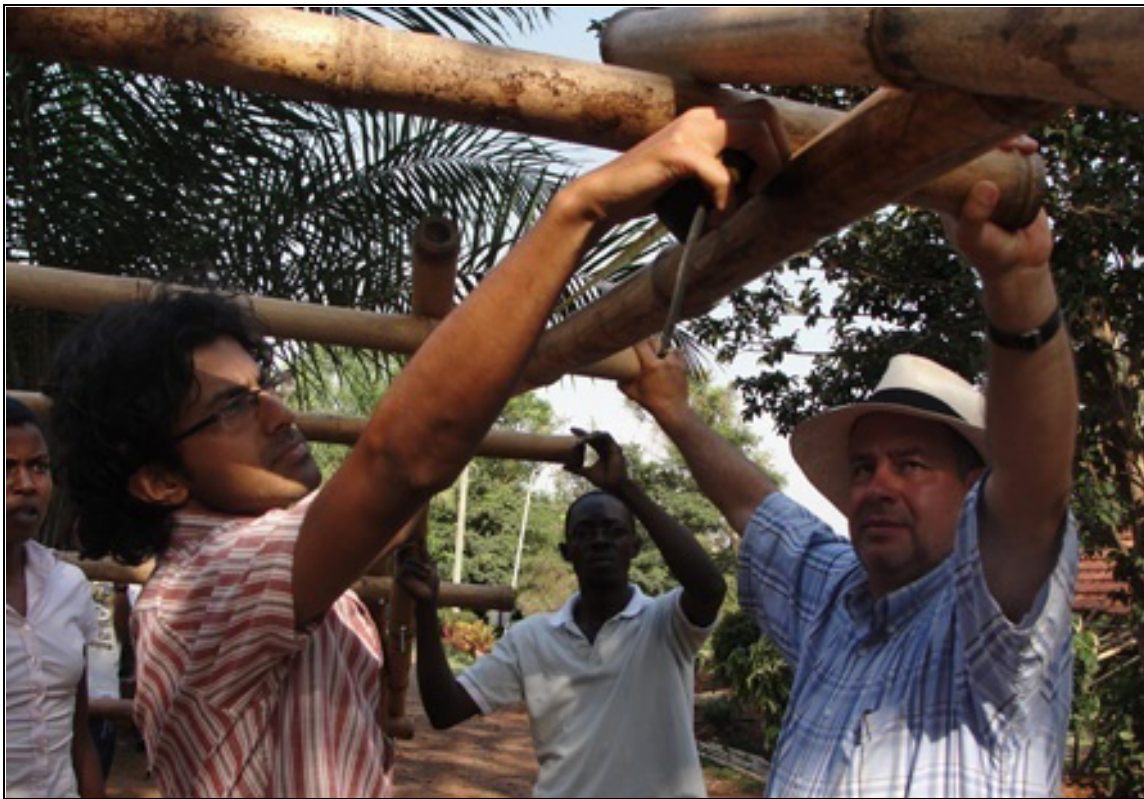
Picture 2: Architects Juan Carlos and Nripal Adhikary teaching trainees about bamboo joints
