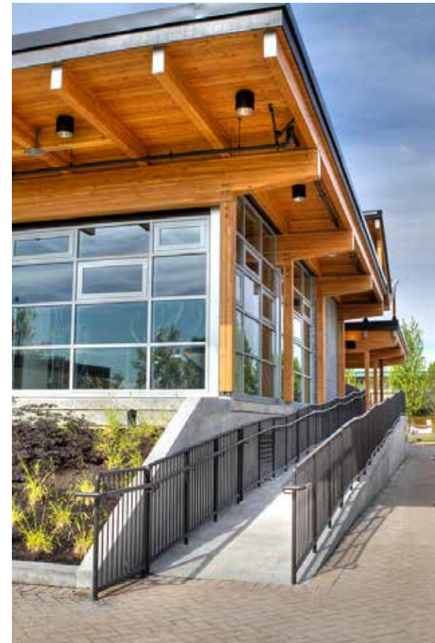
Straight Run for Wheelchair Ramp is preferred to a ramp that switches back 180 degrees.
