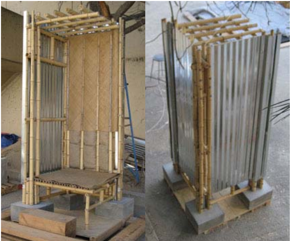
Figure 5.12 A full-scale section prototype constructed to test the feasibility of the proposed low cost housing solution. Source: Photographs by Author.
