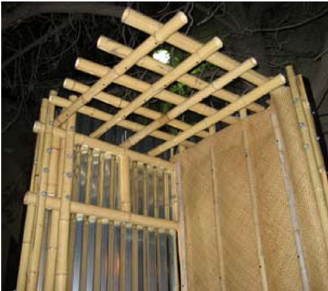
Figure 5.13 Upper portion of the prototype showing parts of the structural system, a partial roof system and the internal wall covering. Source: Photograph by Author.
