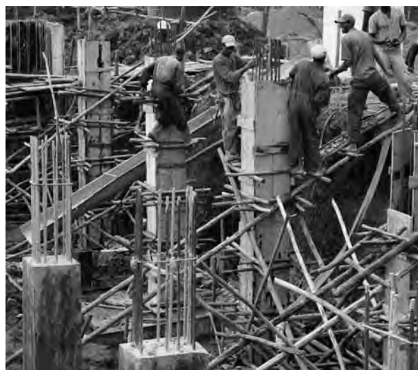
Figure 31: Labourers building the foundations for Lideta condominiums Lideta, Addis Ababa. © UN-HABITAT/ Katherine Hegab
