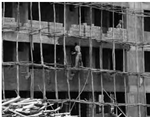
Figure 28: Workman applying plaster to the first-storey of a condominium block. Bole Summit, Addis Ababa. © UN-HABITAT/ Katherine Hegab
