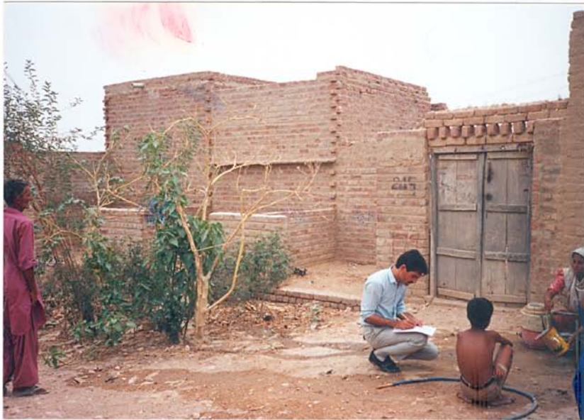
Good walls but no roof
