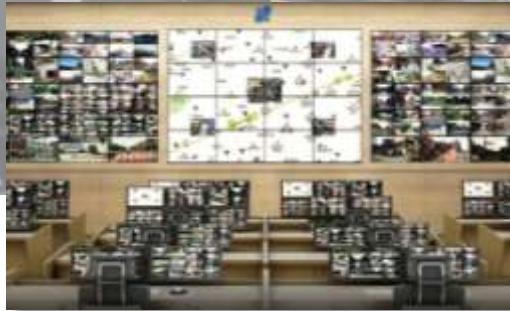
• Command Control Center
