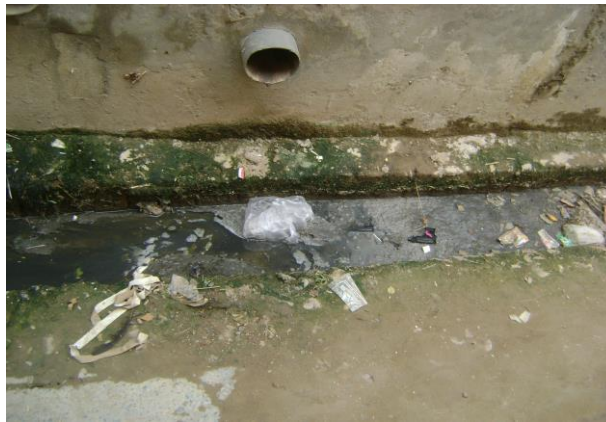
Fig 4.6: Open sewers in badar colony
