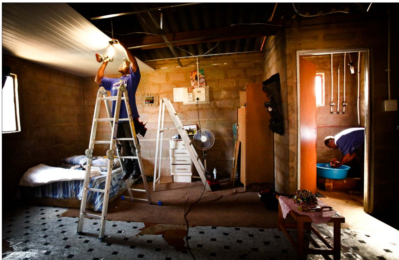
A CFL efficient light bulb is fitted, while the ceiling boards are still in the process of being installed on the fitted metal framework. In the bathroom another worker is washing his hands using the solar-heated hot water. Safe wiring and plumbing can also be seen.
