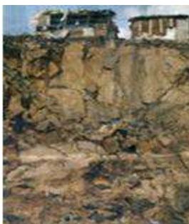
Figure 28: Encroached hill marred by landslides at Andheri
