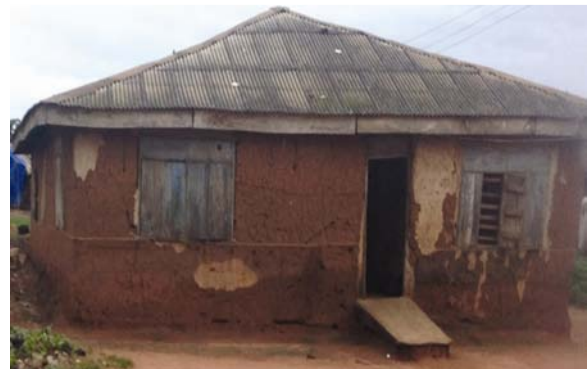
Fig. 2—An earth building in Ota with its protective cement coating on wall already falling off
