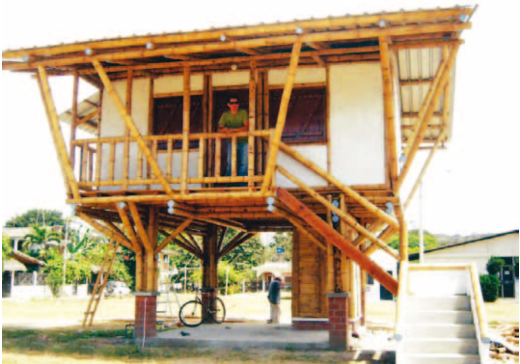
Improved bamboo home prototype built in Olon community, Santa Elena province, Ecuador in 2011. © INBAR LAC.
