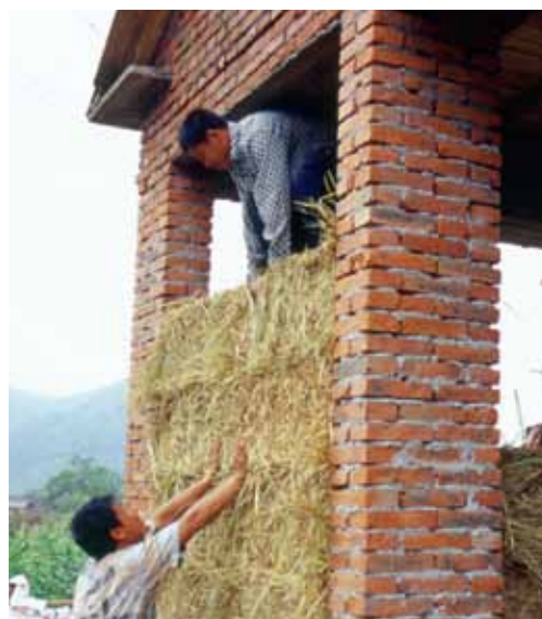
Stacking straw bales between brick columns, Heilongjiang, China. © Kelly Lerner, One World Design Architecture.
