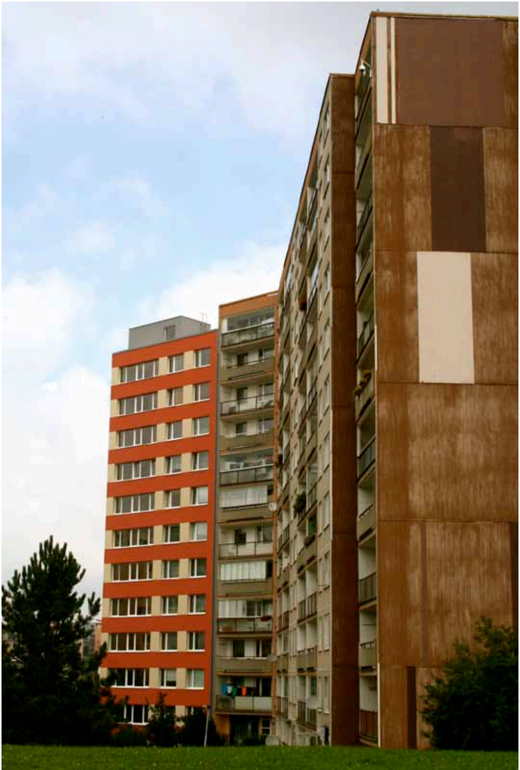
Post-war multi-storied housing in the Czech Republic under environmental retrofitting. © Matthew French, UN-Habitat.
