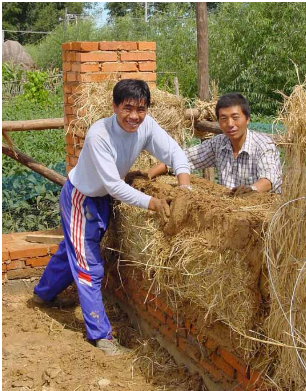
Stacking strawbale walls with earthen mortar, Jilin, China. © Kelly Lerner, One World Design Architecture.
