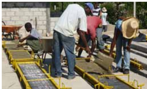
A mobile vibrator forms the panels (above). Alternatively panels are produced by hand (below). © Ecosur.
