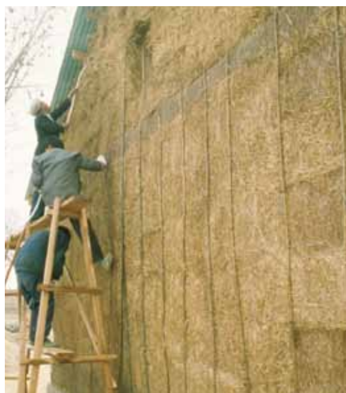
First strawbale school in China under construction, Hebei 1998. © Kelly Lerner, One World Design Architecture.
