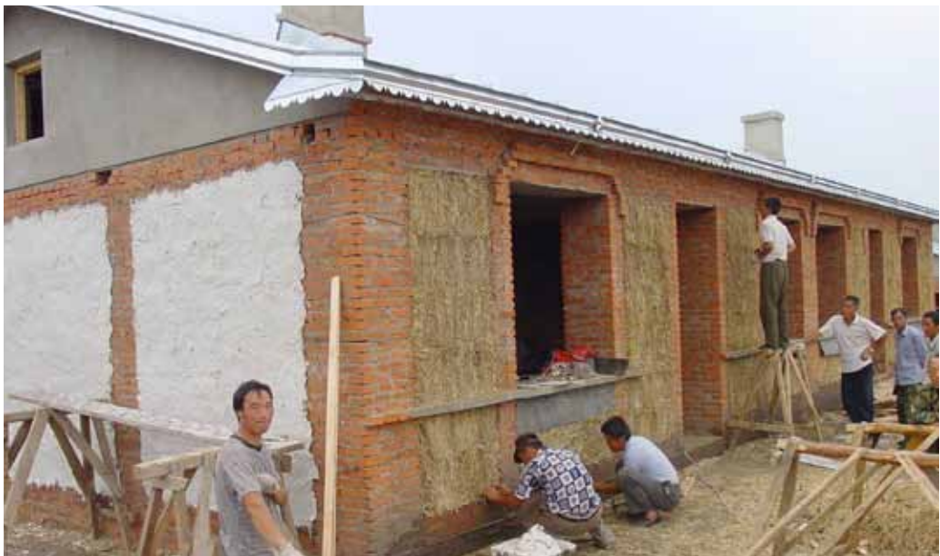
Strawbale house with brick frame under construction. © Kelly Lerner, One World Design Architecture.
