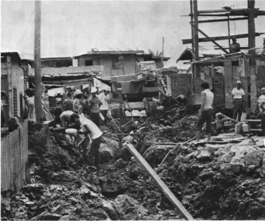
The water system in the Tondo sites-and-services project, Manila, has been a self-help scheme.
