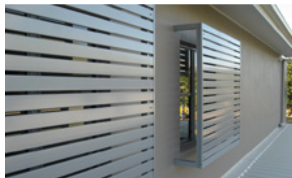
Figure 3-64 Poorly executed privacy screens. These block outlook, sunlight and daylight to windows and reduce amenity of room.
