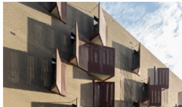
Figure 3-65 Angled privacy screens direct views away from the side boundary. They could also include bay windows
