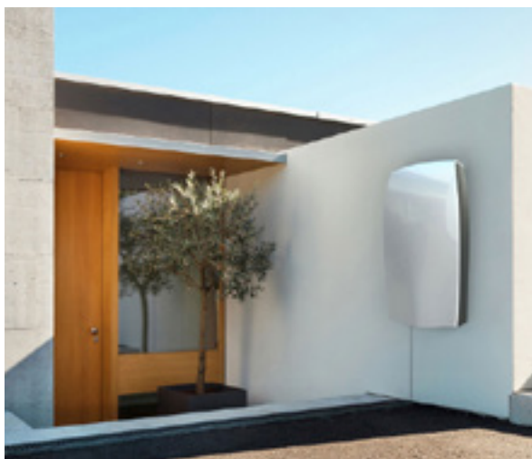
Figure 3-99 Battery storage saves energy generated during the day for use in the evening
