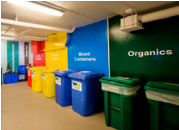
Figure 3-110 Well designed, easily accessible and clean waste and recycling rooms improve the collection and management of household waste
