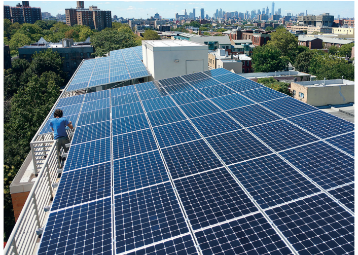
A rooftop solar PV array on a multifamily apartment building in Brooklyn, New York. Photo credit Bright Power, Inc.
