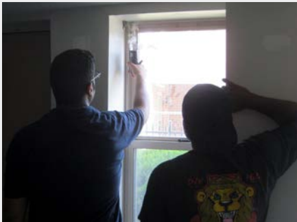
Combined with blower-door testing, smoke pens helped PHIHA staff determine the most important locations to air seal in typical units.
