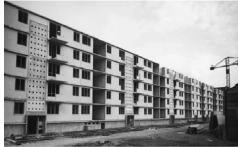
Image 3: Social housing construction based on the Camus system of large panel, pre-fabricated construction in Nanterre. Source: Bullock (2009)
