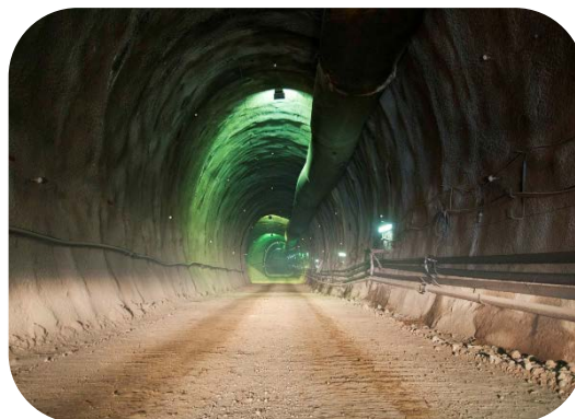
Example of the proposed combined line infrastructure tunnel; includes sewer line, electricity lines, fibre optic cables and water lines
