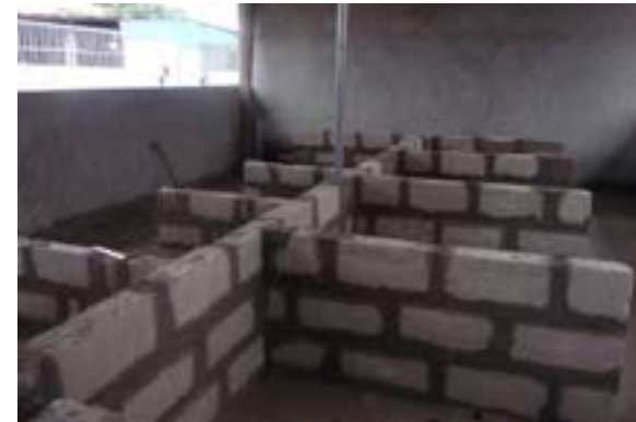
A composting area built to improve solid waste management practices in Accra.
