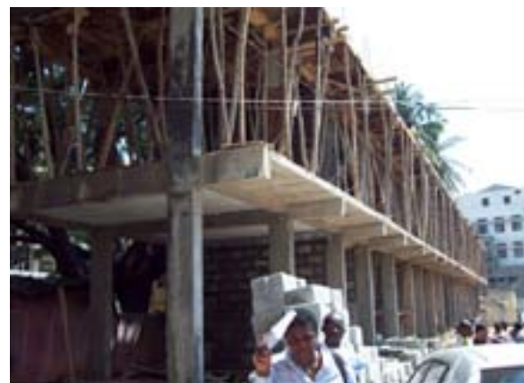
CHF/MM assisted BBMP redevelop a slum in Bangalore. This new structure will house 25 households with water and sanitation in each unit.
