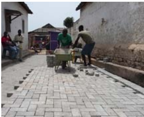
Almost 1,000 square feet of alley have been paved in the Ga Mashie area.
