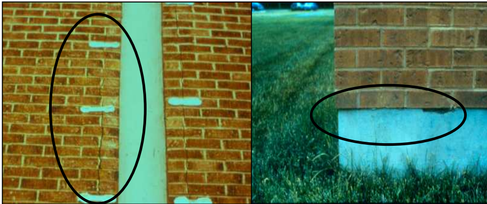
Figure 4.6 – Two Examples of Cracking Induced by Volume Changes
