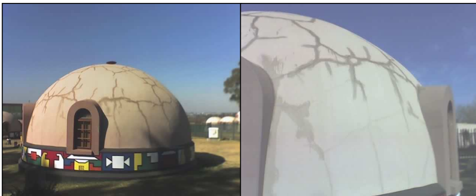
Figure 4.12 – Cracks Patterns around Openings at the Sparrow Aids Village
