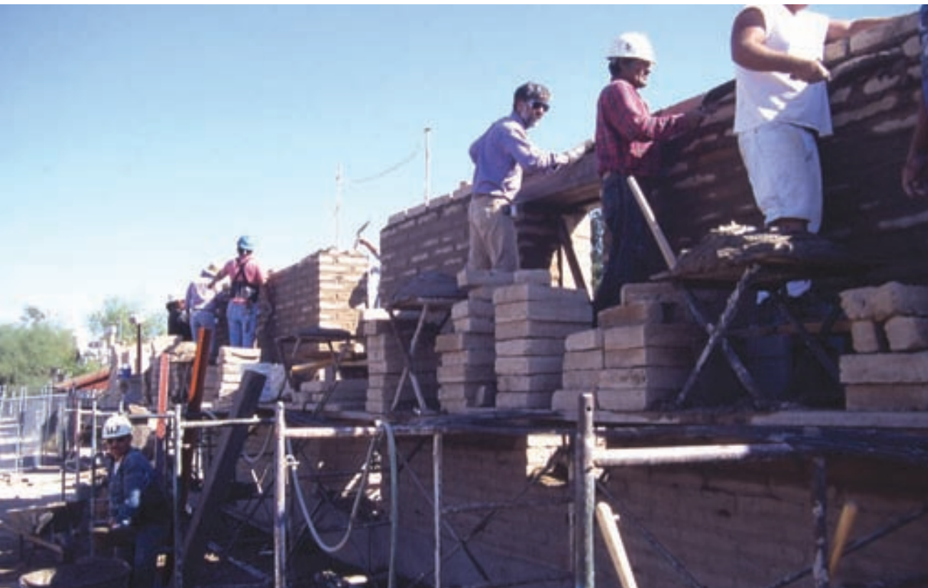
Adobe wall under construction in Tucson, Arizona, illustrating the amount of labor required to raise a wall. Photo: B. Vint
