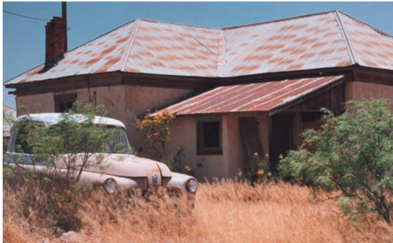
New Mexican ranch house with corrugated galvanized iron roofing. This metal roof is approximately 50 years old, and is still effective. Photo: B. Vint
