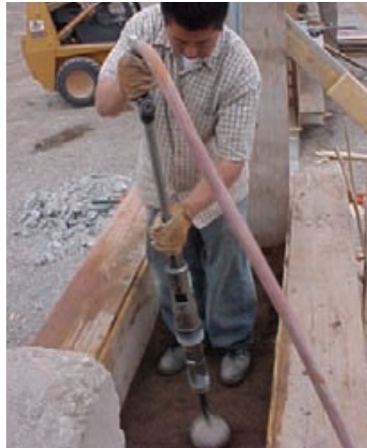
UA design/build student ramming earth with a pneumatic tamping machine known as a Jumping Jack. Note custom lumber formwork. Photo courtesy of M. Hardin
