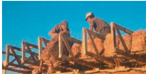
In the Colonia Anapra straw bale house, bales are used as roof insulation between palette trusses. Photo: C. Wanek
