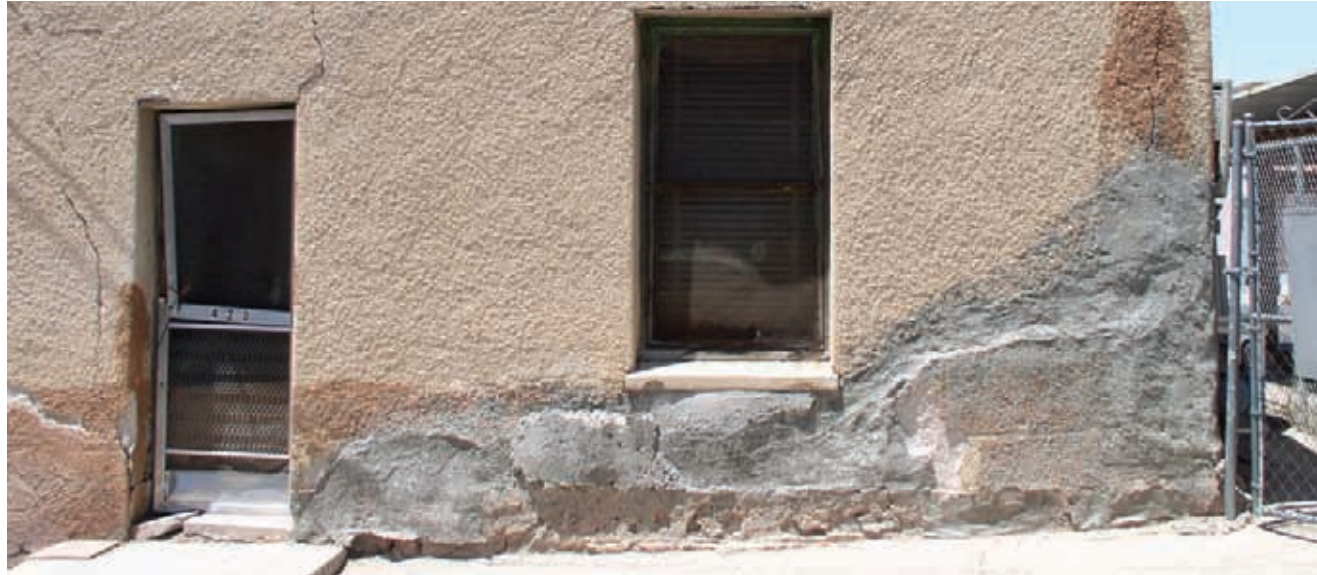
Effect of cement repairs to adobe: moisture from foundation wicks by capillarity through adobe and is unable to escape through cement stucco. Damp adobe is softened and compresses, pushing stucco off wall; water rises ever higher in wall as further cement repairs are made. The correct finish for unstabilized adobe walls is a "breathing" unamended mud or lime and sand plaster that allows the transpiration of moisture vapor. Photo: B. Vint
