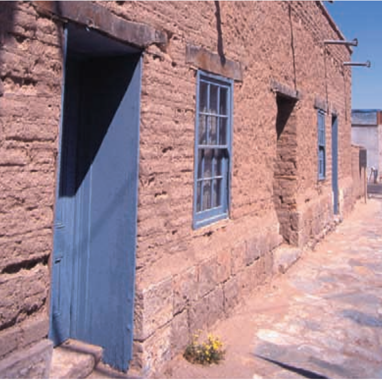
Dressed stone foundation at La Casa Cordova Tucson, AZ. Height of stone above grade protects adobe from splashing of rainwater and isolates wall from rising foundation moisture. Photo: B. Vint
