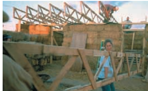
Volunteers carry pallet trusses to be set atop the completed bale walls. The trusses rest on a continuous wood bond beam which ties all the walls together. Photo: C. Waneke
