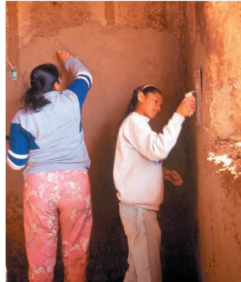
Applying earth plaster to the interior of a straw bale house in Colonia Anapra. Photo: C. Waneke
