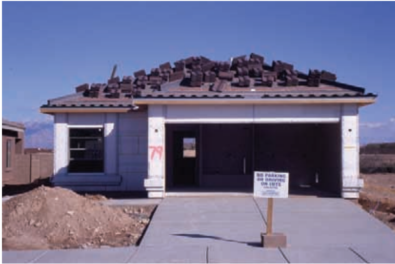
Wood-frame house sheathed in foam awaiting synthetic stucco coating. Glue-on foam moldings seek to provide some differentiation between identical units. Photo: B. Vint
