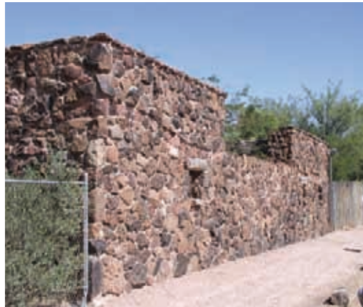
Elder's Center, San Xavier District. Foundation and walls built of volcanic stone. Gibbs & Vint, Architects Photo: B. Vint
