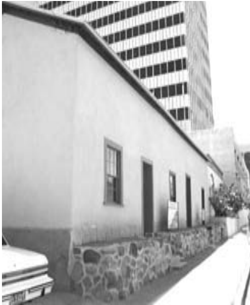
Northwest corner: window and door trim color differentiates individual dwelling units. Photo: P. Briggs
