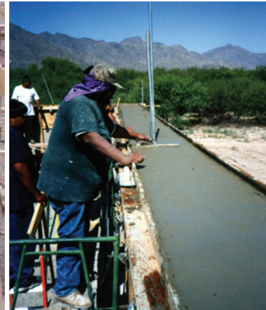
A tribal member smooths the concrete bond beam where the roof assembly will be connected to the earthen walls. Photo courtesy of M. Hardin
