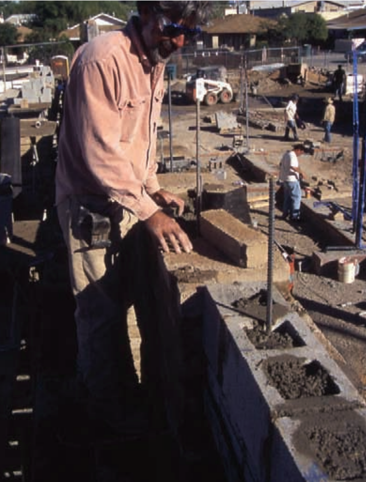
Eric Means, mason and general contractor, installs a reinforced concrete block (CMU) bond beam at roof level of adobe wall. Photo: B. Vint
