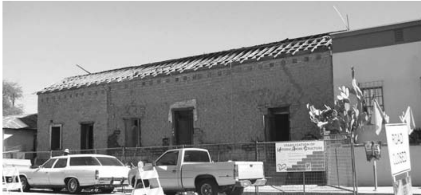
Adobe row house undergoing stabilization. With plaster removed, large joint in adobe wall is evidence how the building evolved over its 130 year history. Photo: C. Neumann
