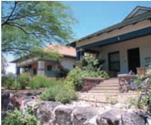
Volcanic basalt used for site retaining wall and foundation early 20th C. bungalow, West University, Tucson AZ Photo: B. Vint
