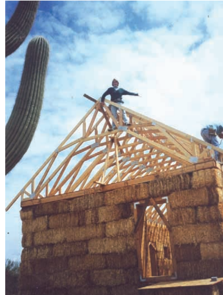
The owner atop prefabricated 2x4 wood trusses which form the gable roof structure. Photo: A. Proczka
