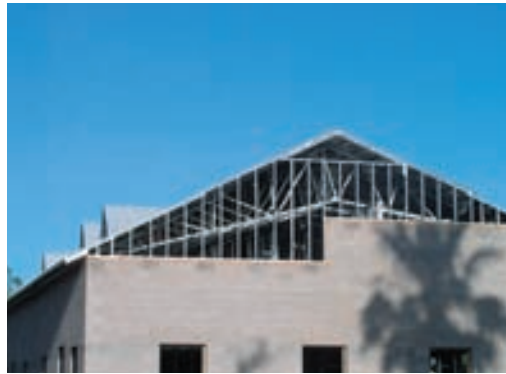
Light gauge steel truss framed roof with metal framing at gable end. Affordable row house under construction in Tucson, AZ. Architect: Joe Comella, City of Tucson Community Services Department. Photo: B. Vint
