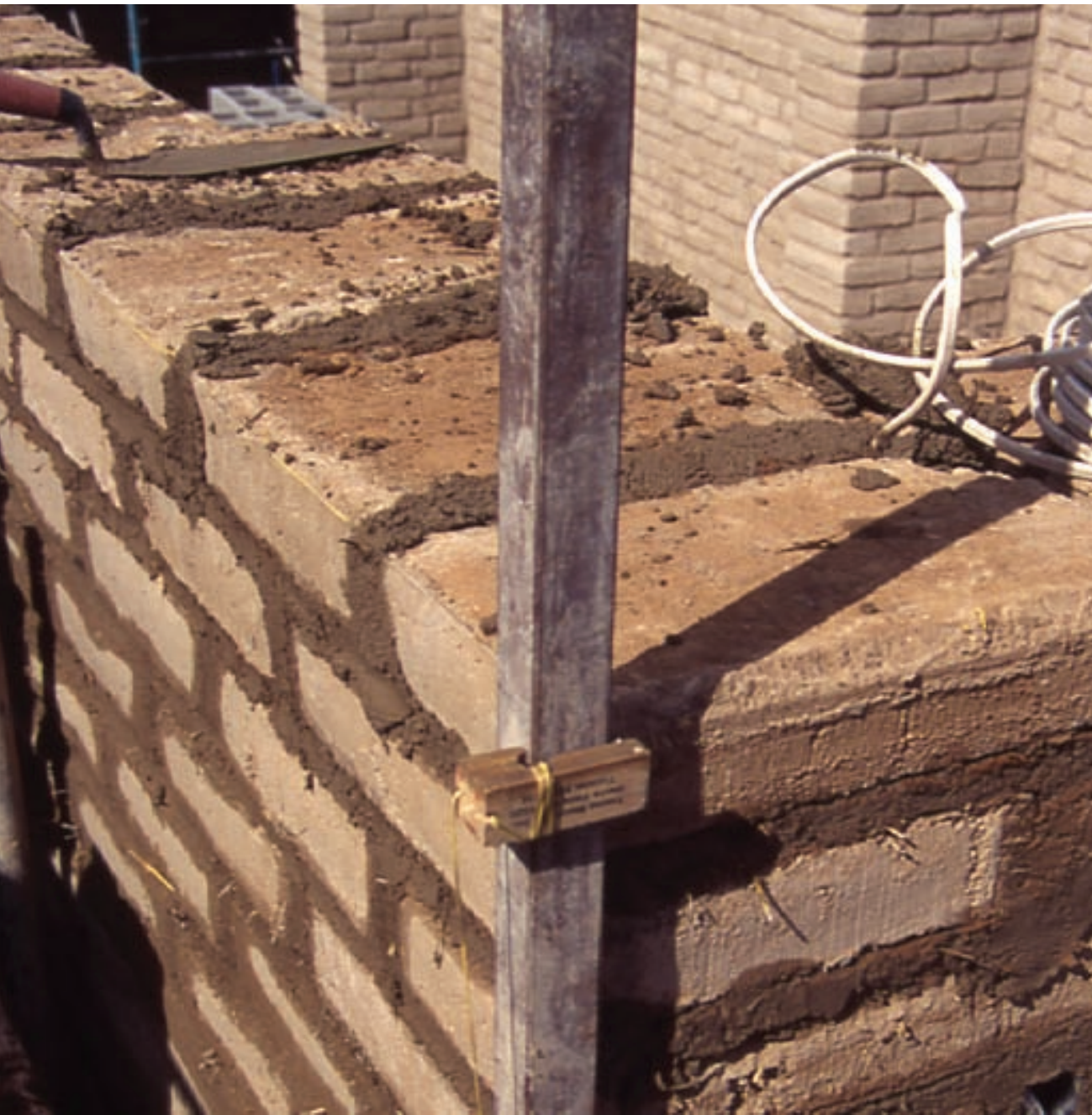
Adobe house under construction Tucson, Arizona. Note mason's corner story pole and electrical wiring being laid in mortar joint so that interior will not have to be furred out. Photo: B. Vint
