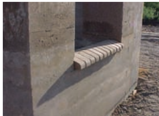
8 Sills protected with tile.
