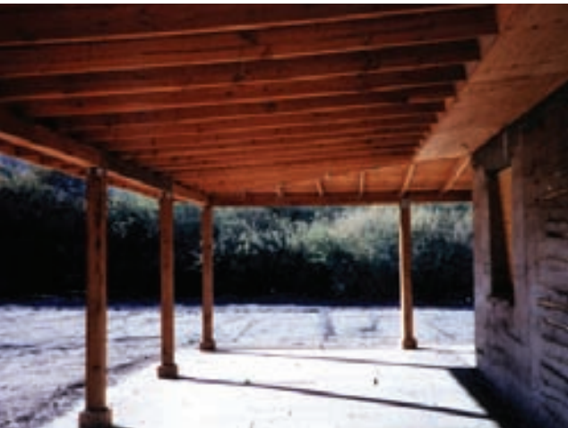
The Della Hughes Family House after rough work (walls and roofing) has been completed. The wide porch which shades the south and west side of the residence aids in passive cooling and provides the family with outdoor living space. Photo courtesy of M. Hardin
