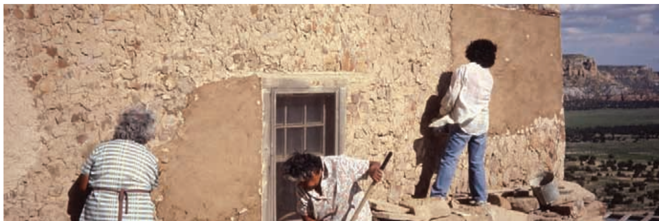
Women of Acoma periodically renew the earthen plaster of the mud and stone walls. Photo: P. Nabokov, by courtesy of the photographer
