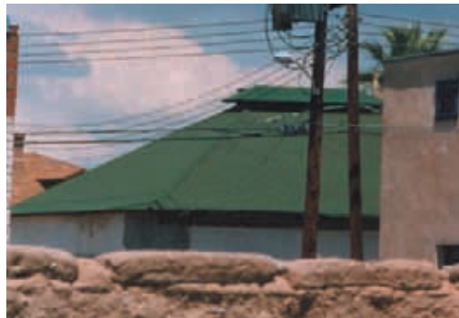
Tucson, AZ: Asphalt roll roofing on the hipped roof of a historic building. Roll roofing is the least expensive and least durable roofing option. Photo: B. Vint
