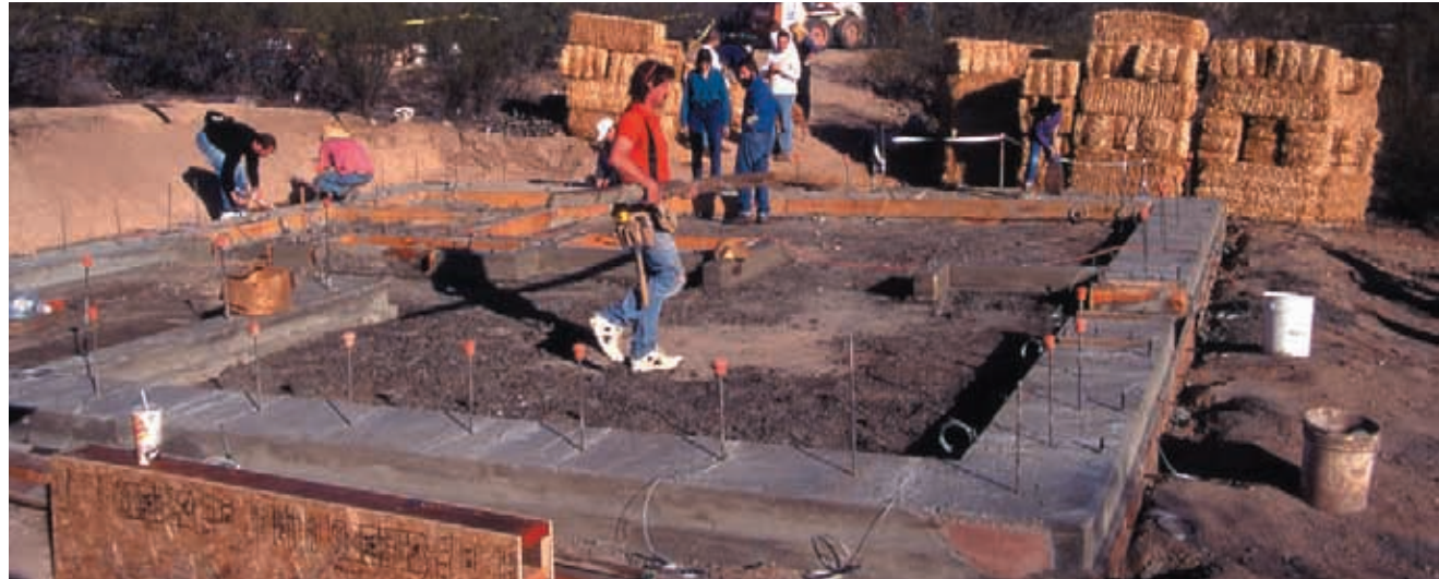
Cast in place foundation for a straw bale house in Tucson, Arizona. Continuous concrete perimeter ties bale walls together and elevates them above ground level to keep them dry. Vertical rebar dowels are used to pin first course of bales to foundation to prevent them from sliding under lateral loads. Floors will be brick laid over sand. Architect: Bob Vint, Tucson. Photo: B. Vint
