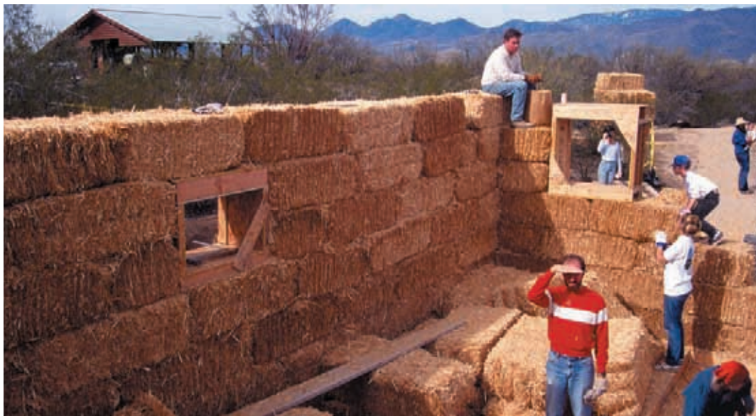
Tucson, AZ: Volunteers place straw bales around a window buck. This one-bedroom house has a modest 676 sf net floor area, but has been enjoyed by the owner since 1997. Design: B. Vint, Architect Photo: B. Vint
