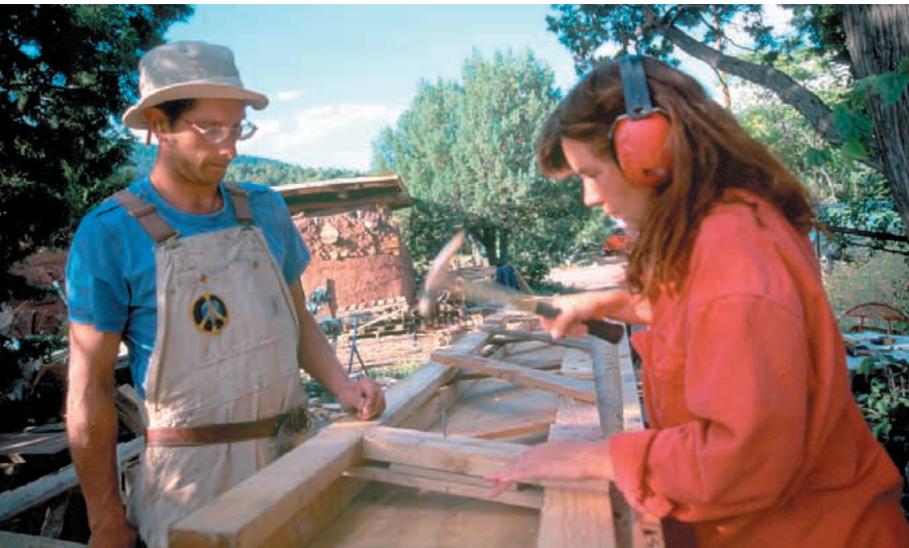
Volunteers build pallet trusses. Wooden pallets are plentiful in Mexican border towns as a result of the maquiladora factories. Re-using pallets not only saves the homeowner material costs, but is environmentally advantageous both for forest preservation and a reduction of carbon dioxide emissions due to reduced trucking of materials. Photo: C. Wanek
