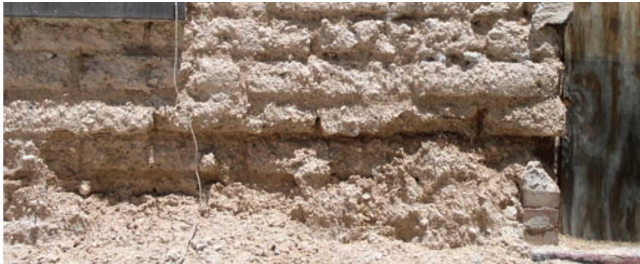
Long-term effect of cement on unstabilized adobe: deterioration of wall base due to rising dampness trapped by cement. Walls eroded at the base are prone to collapse, when dampened during the rainy season, for they are weakened exactly where the accumulated weight of the wall above is greatest. Photo: B. Vint
