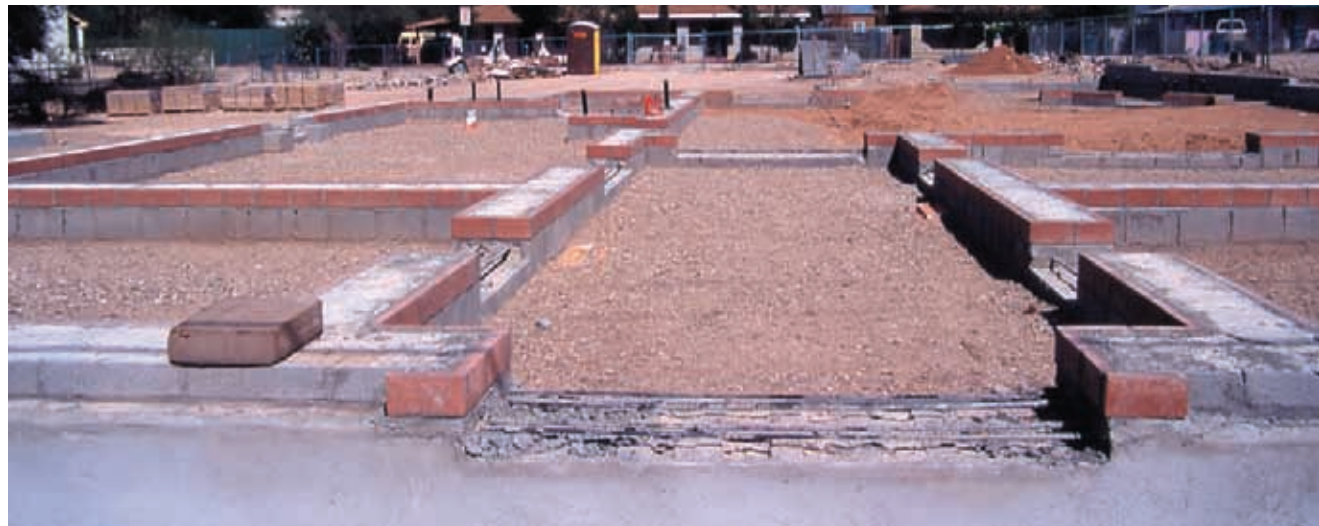
Foundation stem wall for an adobe house in Tucson, Arizona. The stem wall is solid grouted CMU with horizontal and vertical reinforcing. It is supported on a reinforced concrete footing approximately 12 inches thick, placed at two feet below grade. The footing and stem wall together constitute the foundation system. Floors are to be colored concrete slabs on grade. Architect: Bob Vint, Tucson. Photo: B. Vint
