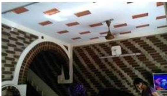
Fig -12: exposed bricks and filler slabs
