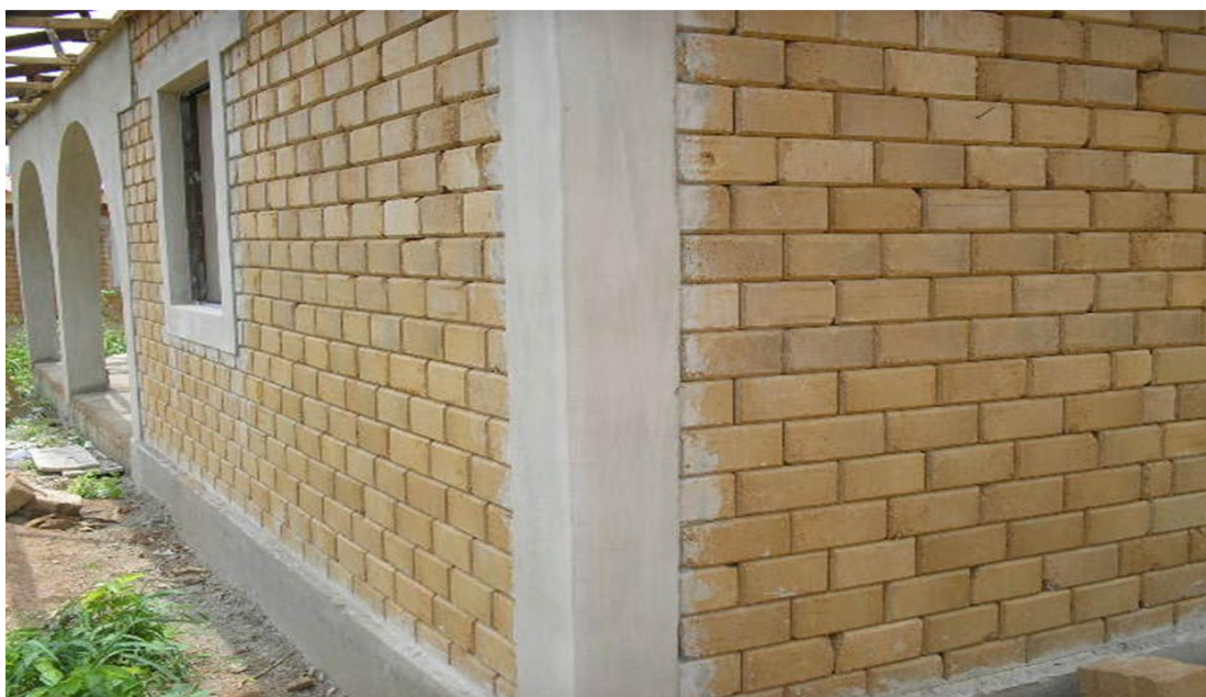
Figure 3: Interlocking Masonry at the Finishing Stage of a Housing Project. Source: Field survey, 2007
