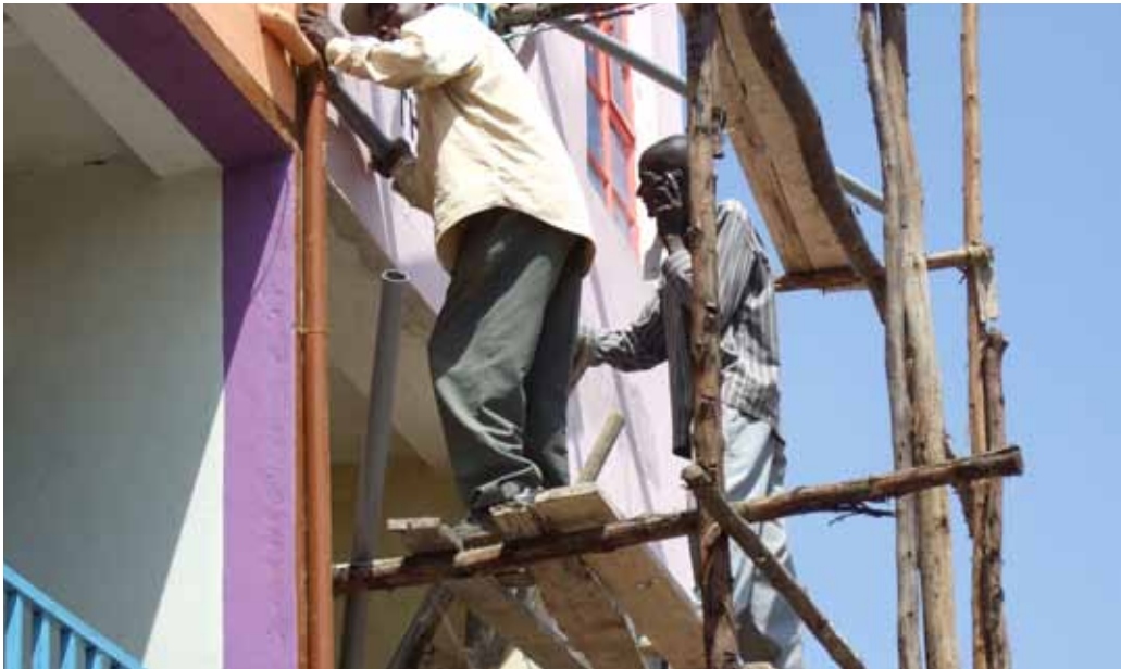
Training should target safety in construction, as job-related accidents are common among poor construction workers in developing countries . © Oleg Golubchikov/UN-Habitat.
