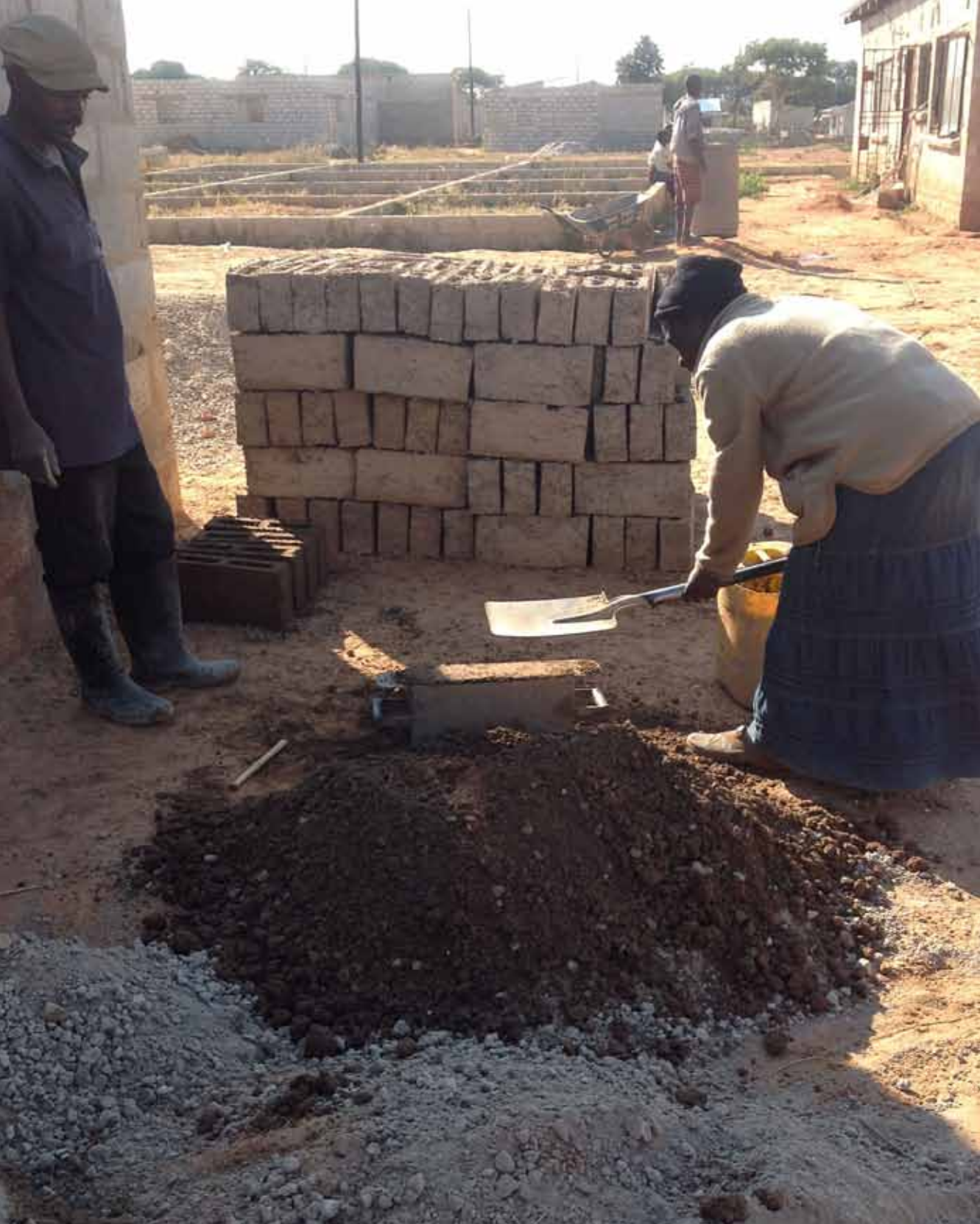
Construction work by community members in an informal area of Lusaka, Zambia. © Matthew French/UN-Habitat.
