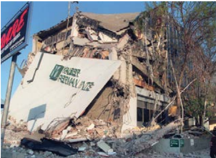
Concrete structures, like this Kaiser Permanente building, collapsed when exposed to the ground movements experienced in the 1994 Northridge earthquake. (USGS)
