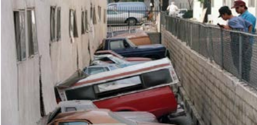
The collapsed Northridge Meadows apartment buildings were a striking example of how soft-story structures can fail in an earthquake. (USGS)
