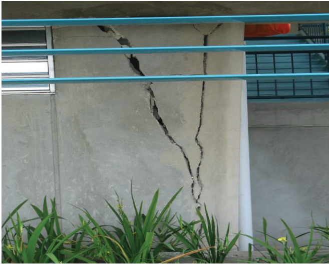
Figure 6: Wall failure due to Diagonal Tension
