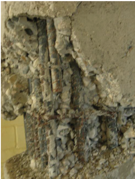
Figure 8: Close-up of failure zone
