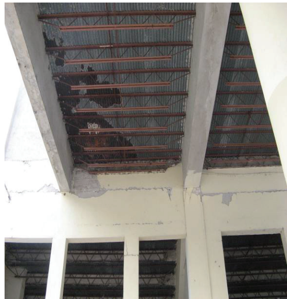
Figure 10(b): Close-up of failure zone
