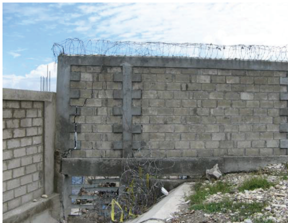
Figure 14: Failure of Masonry Wall
