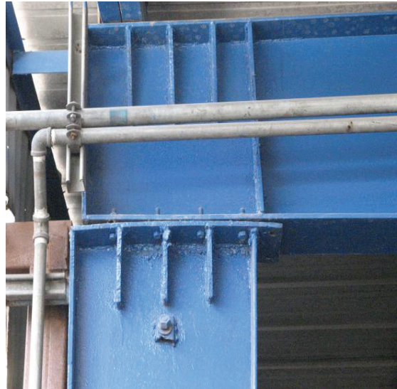
Figure 13: Deformed Joint in Steel Frame
