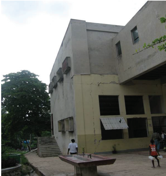
Figure 10(a): Failure of Wall in Auditorium
