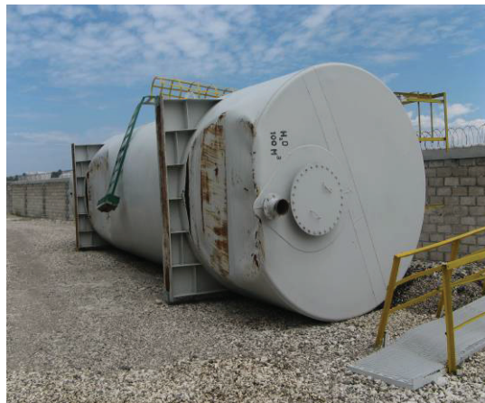
Figure 15: Overturned Fuel Storage Tank
