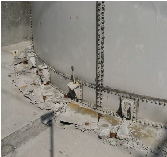
Figure 12: Base Attachment Failure
