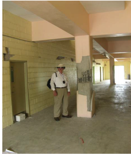
Figure 7: Column Failure at Mid-Height
