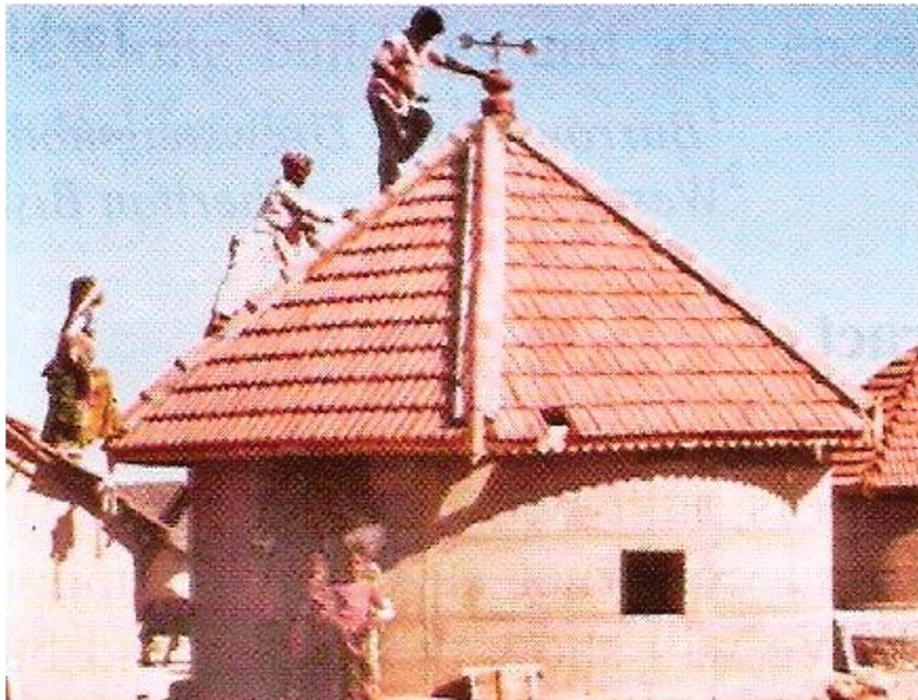
Figure 4: Circular house under construction in 2001 Kutch earthquake rehabilitation exercise. Source: Kotak (2007, p. 71).
