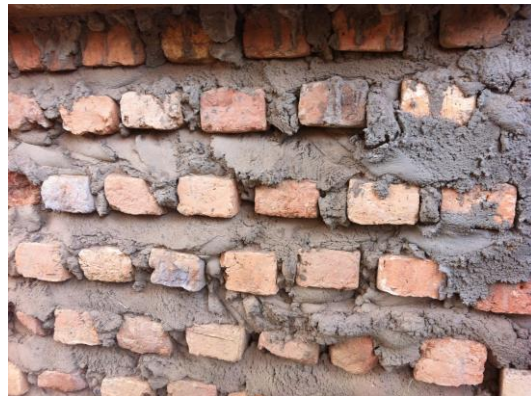
Image 2: Excessive mortar joints contribute to waste associated with brick construction in Uganda.
