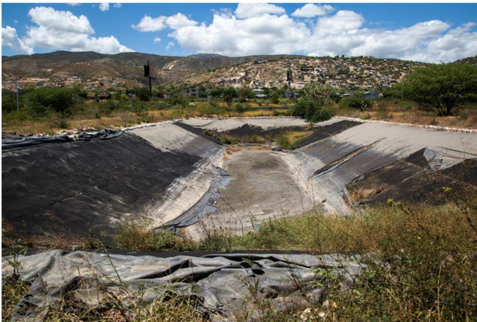
Since 2013, the $2.1 million sewage treatment plant at Titanyen has been closed. The lining of one of the disinfecting basins developed massive bubbles due to an engineering defect. Marie Arago for NPR
