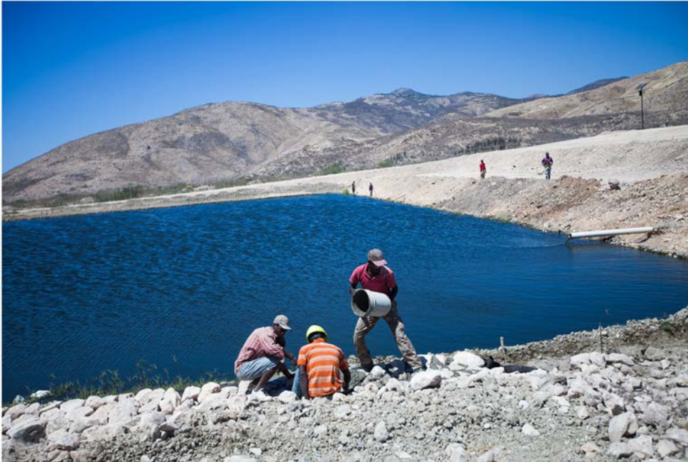
The open-air sewage treatment plant at Morne a Cabrit is the only such facility operating in Haiti. John W. Poole/NPR
