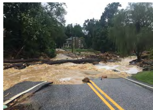
Labor Day 2018 Flooding, Kreutz Creek Road (Hellam Township)- YCPC Photo
