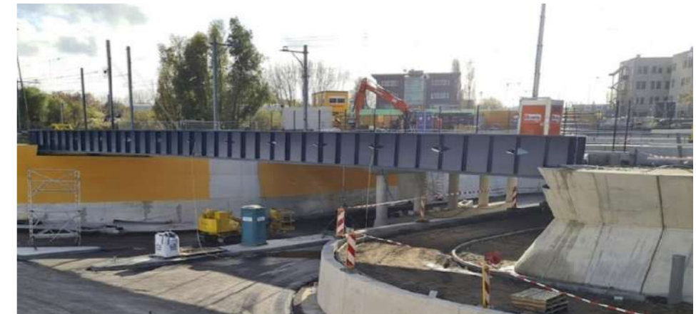
Here the circular concrete mixture produced by Rutte Group with the help of SmartCrusher technology is used in a reinforced concrete component that separates the road from the cycle path. Source: slimbreker.nl, 2022
