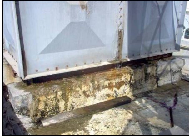
Figure 6. Damaged Water Tanks
