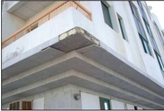
Figure 8. Falling of External Marble Cladding
