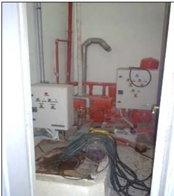
Figure 10. Congested Pump Room
