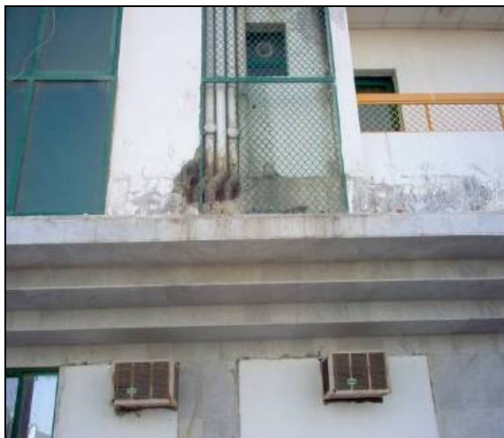
Figure 9. Concealed Sanitary Pipes
