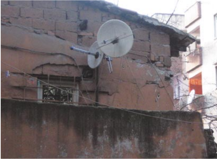
Damaged terrace close-up
