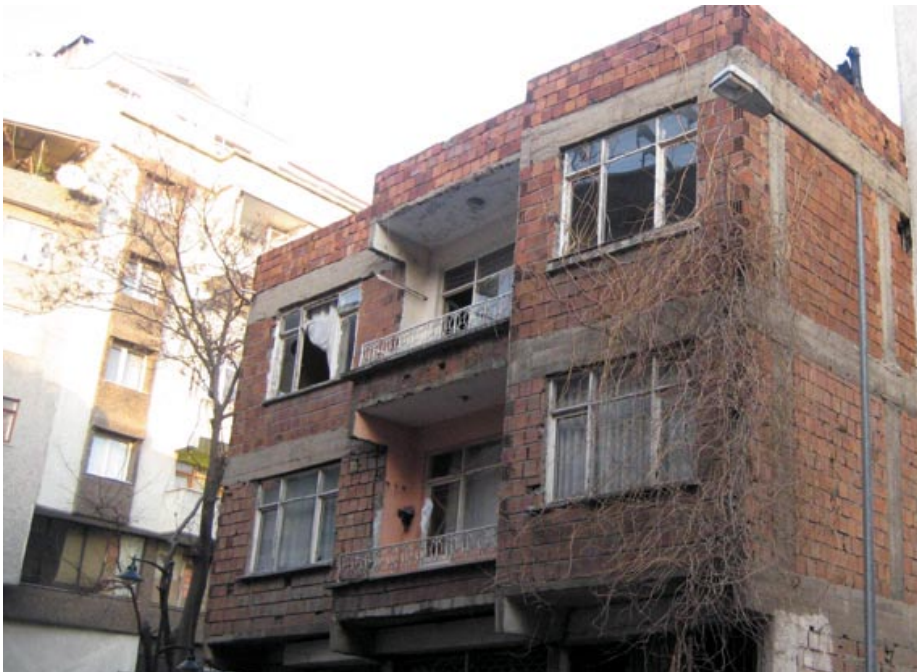
Old and deteriorating building
