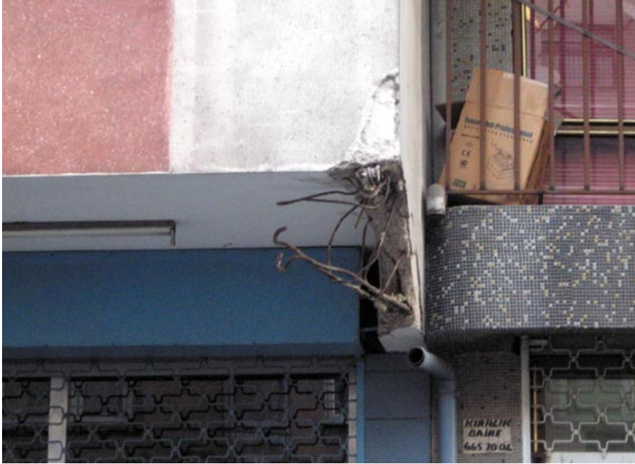
Exposed rebar close-up
