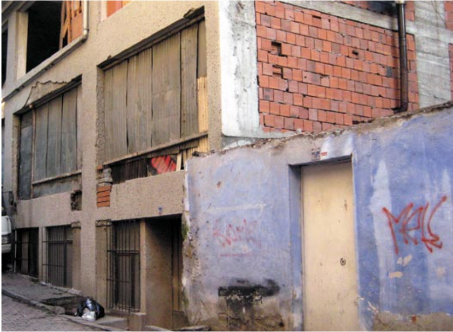
Building in disrepair
