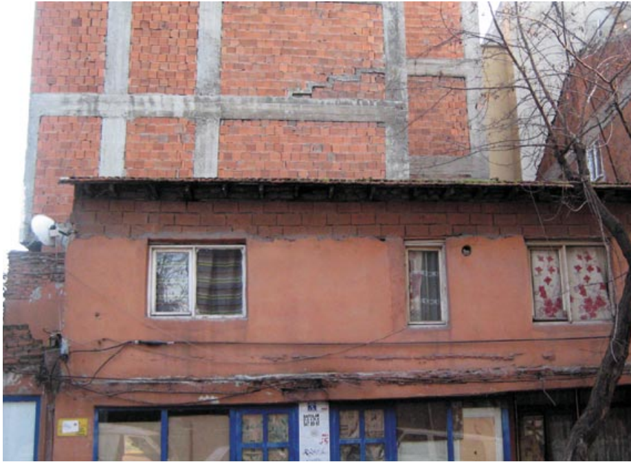
Exposed cables on building exterior
