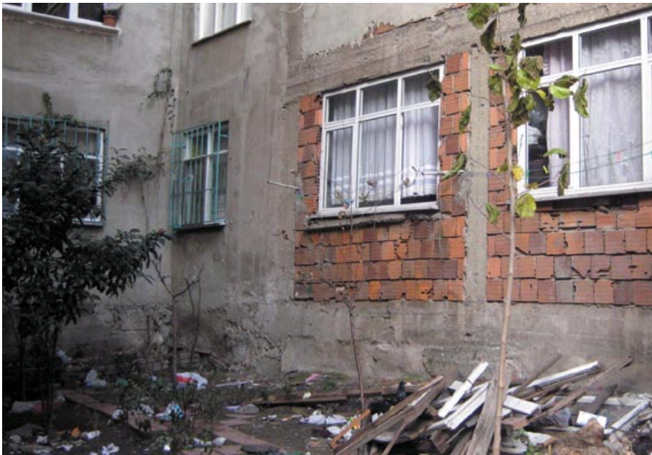
Exposed brick and construction debris
