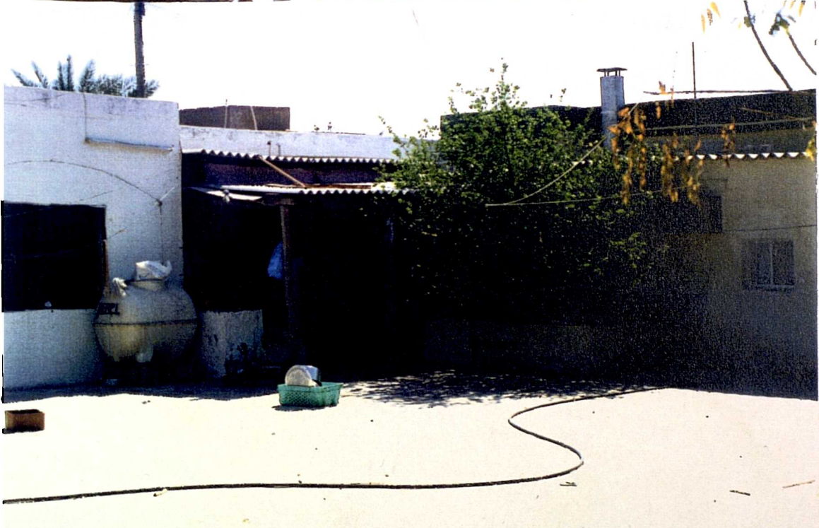
Plates 6.7. and 6.8. The deterioration of reinforced concrete slab forced the user of this low-cost house to abandon his house and occupy the extensions built of asbestos.
