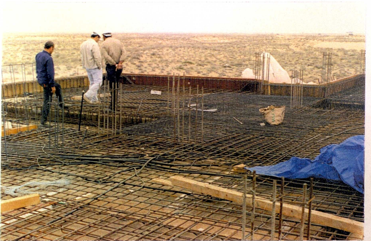
Plates 6.4. The steel work for roof slab of low-cost house under construction
