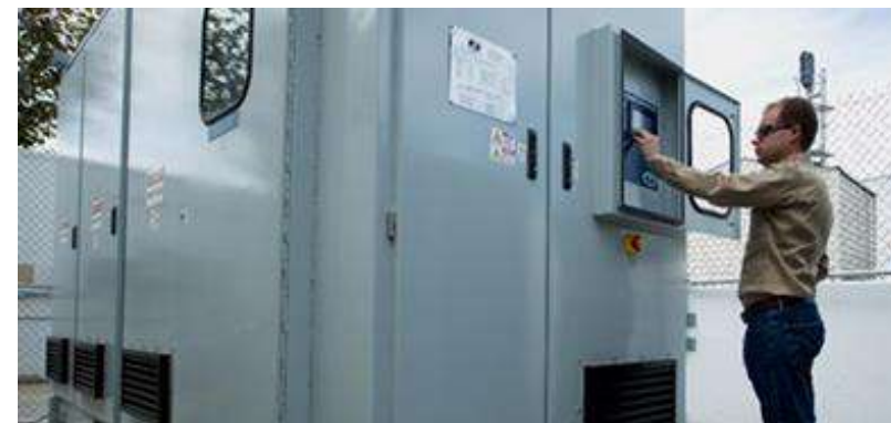
Building Energy Storage Systems Source: https://www.sce.com/safety/bess
