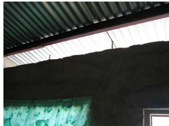
Fig. 11 Ventilation seen from inside, Cabuyao, 2007-04-25
