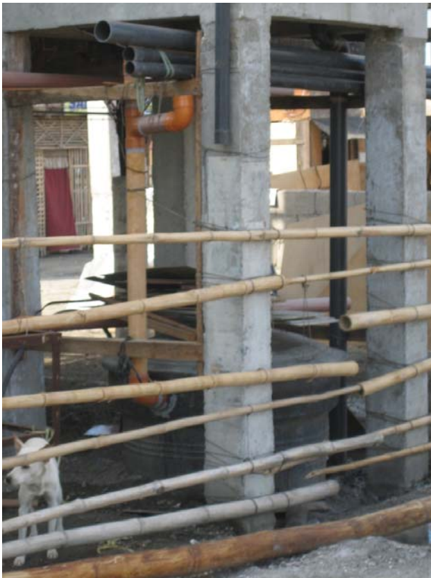
Fig. 31 The septic tank, Sanagmana, 2007-04-28
