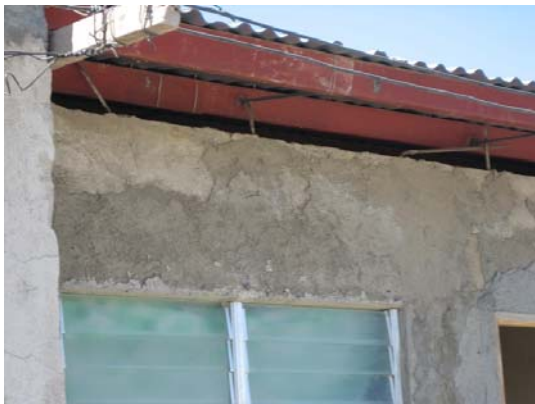
Fig. 10 Ventilation seen from outside, Cabuyao, 2007-04-25
