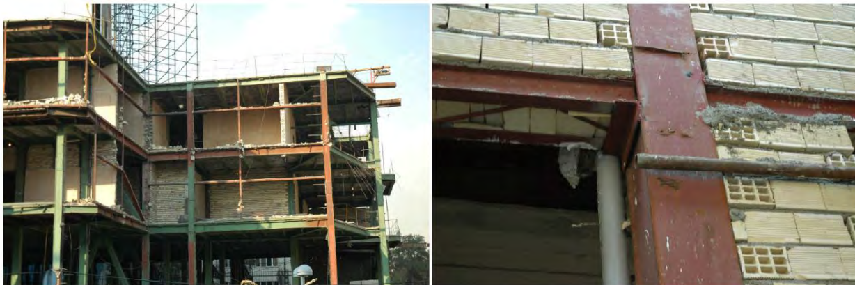
Figure 2: Low building quality in Iran.
