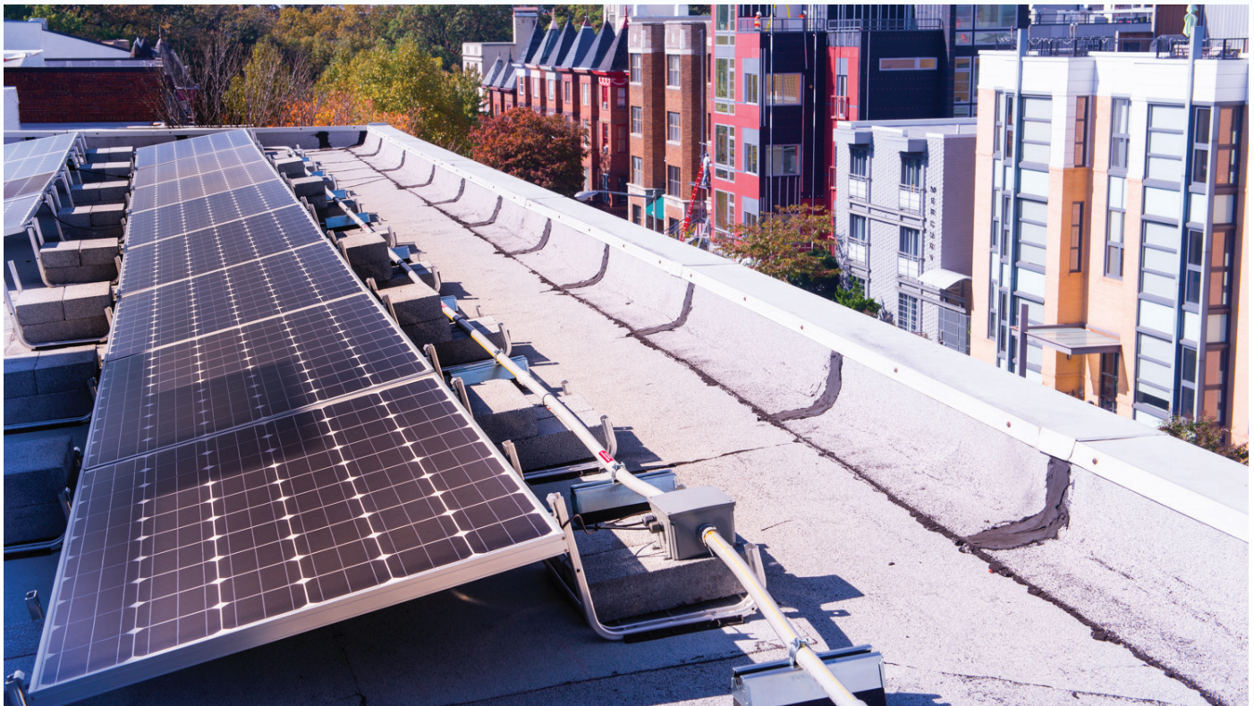
Solar array installed by NHT-Enterprise at St. Dennis Apartments, Washington, D.C.
