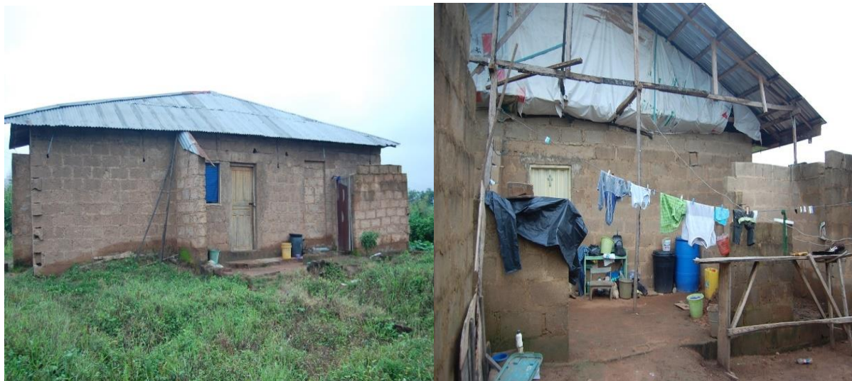
Figure 2. Incomplete houses occupied
