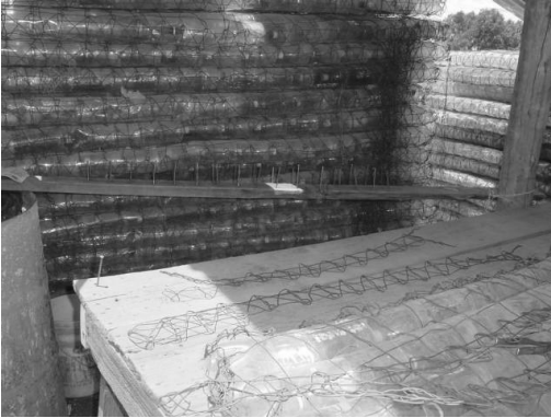
Figure 3: Construction process of PET modules. Perimeter steel frame and wire enclose of bottles.
